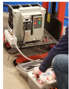
Secondary Injection Testing
