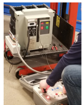
Secondary Injection Testing
